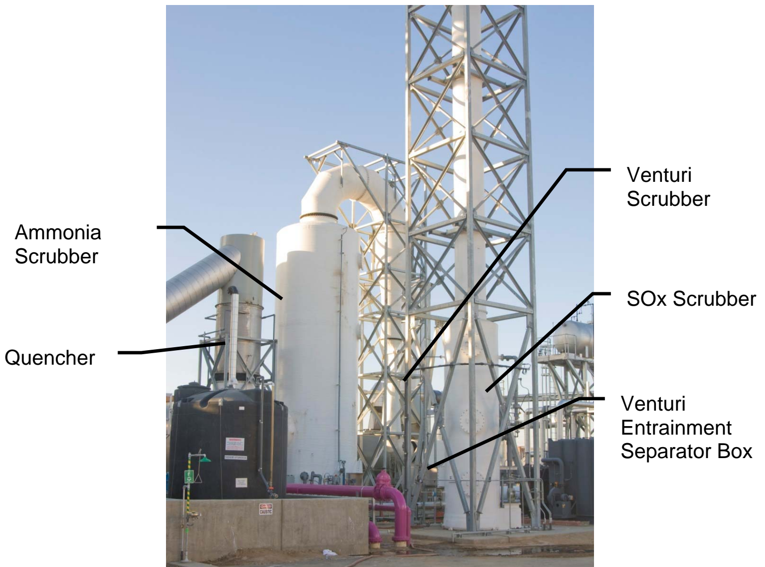
Figure 1: Sludge Dryer Wet Scrubber System
